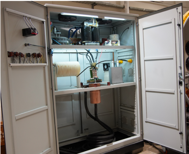
Figure 6: 200 kHz, 10 kV Oscillator Unit.
