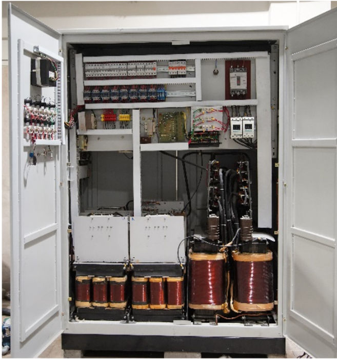
Figure 5: 10 kV/80 kW Silicon-Controlled Rectifier (SCR).
